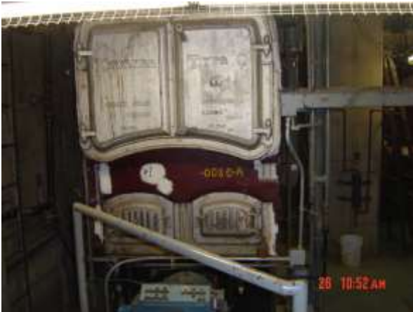
Typical Old Highrise Boiler
