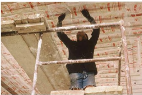
FIGURE 8.6 Inadequate worker protection during a large overhead paint stripping project. Depending on exposure, this worker should be wearing protective clothing, long chemical-resistant gloves and a respirator; and should also be protected against falls.
