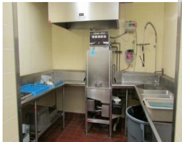
Commercial Kitchen Wash Sink and Oven
