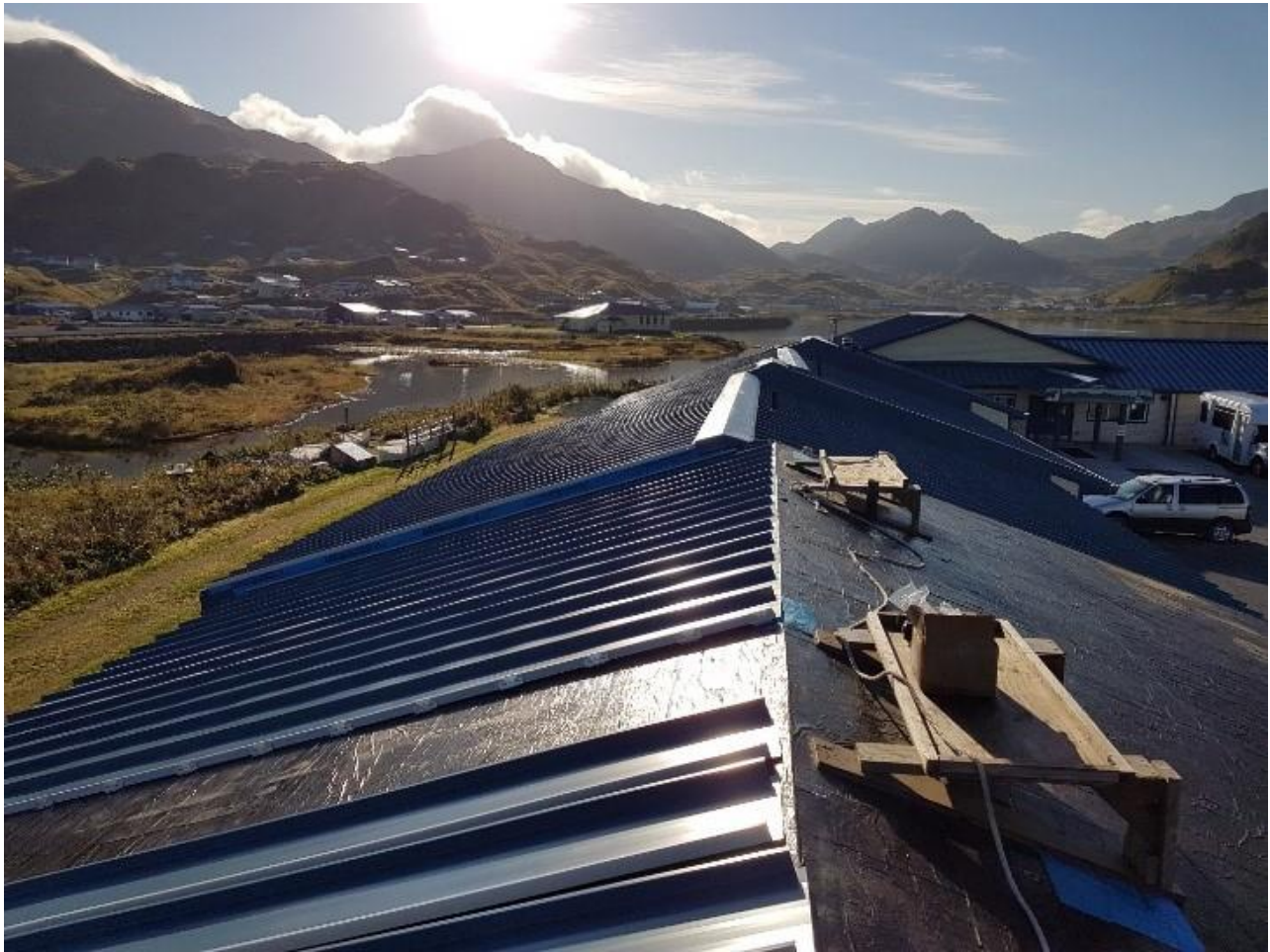
Figure 7: Installation of a new roof on the Unalaska Senior Center in Unalaska.
