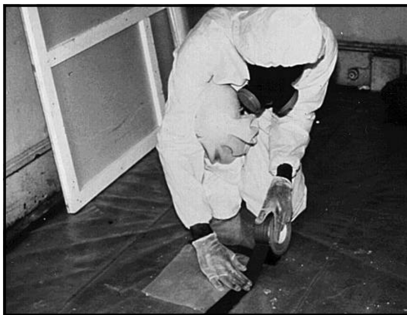
Figure 14.7 Plastic Sheeting Should Be Repaired as Part of Daily Cleanup.
