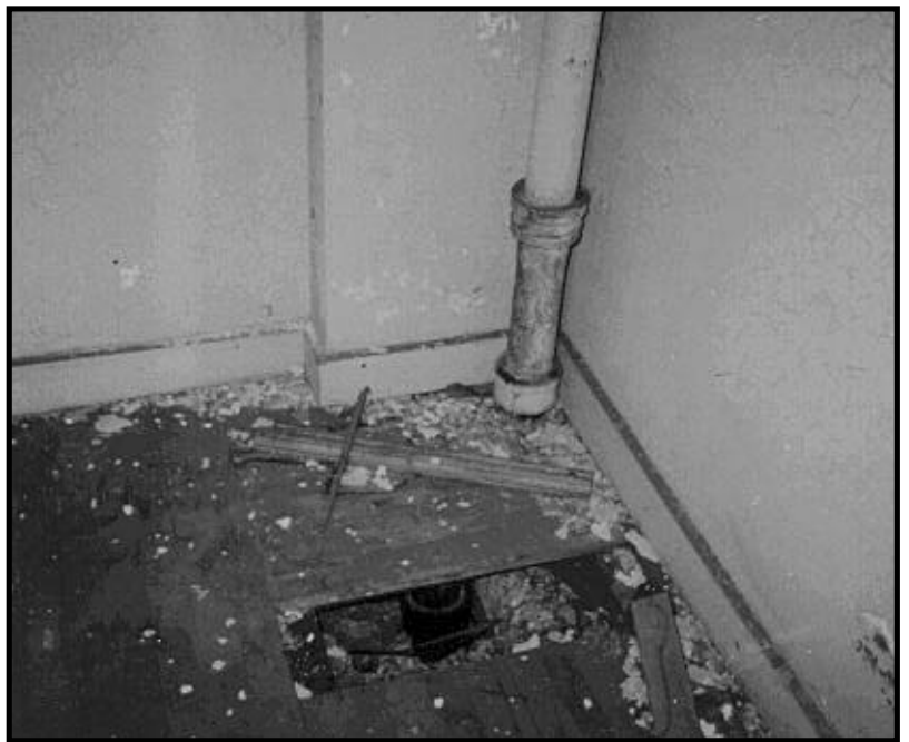
Figure 14.6 Precleaning Is Needed in Areas Where Contamination and Deterioration Are High.
