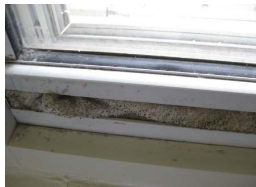
Picture 2: Unit 133. This appeared to be a moldy towel in the window frame. The dirt and chipped paint indicated that the contractor had not cleaned or encapsulated the window frame as required.
