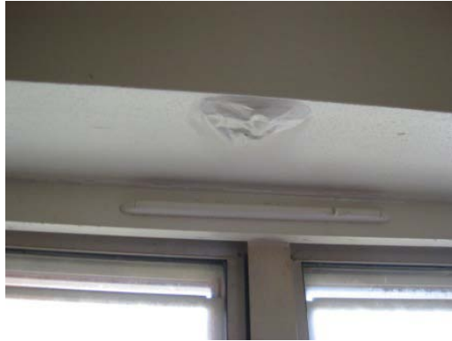
Picture 5: Unit 48. This appeared to be a large paint bubble.
