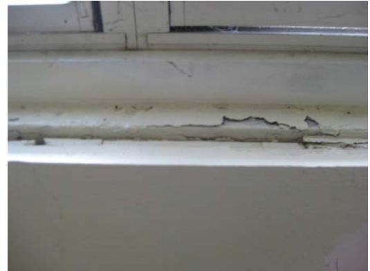
Picture 6: Unit 48. The chipped paint indicated that the contractor had not cleaned or encapsulated the window frame as required.
