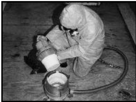
Figure 11.16e Wash or Replace Coarse Prefilters if Necessary.
