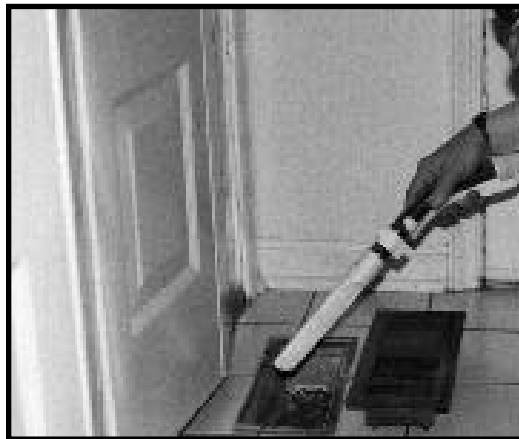
b. Vacuum Accessible Parts of Duct Opening.
