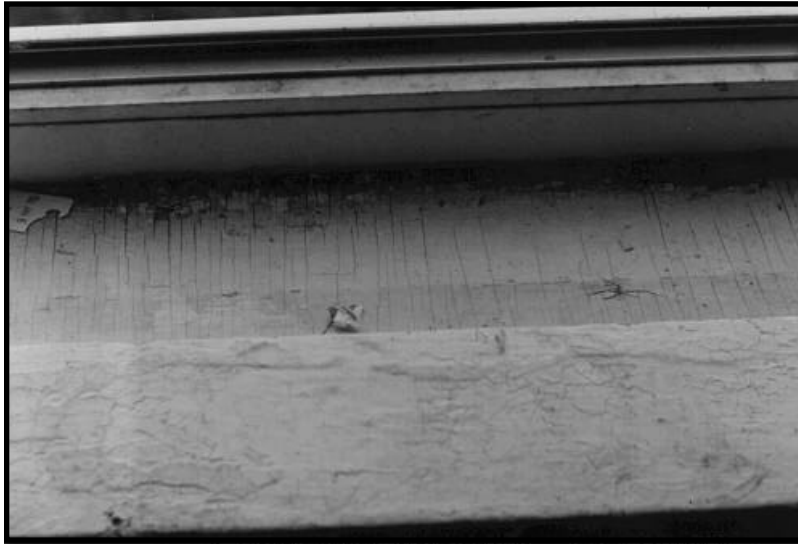
Figure 11.14a Turning a Window Sill and Trough Into a Smooth and Cleanable Surface (before treatment).
